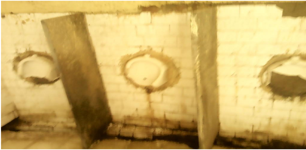
Boys toilet in bad shape in government high school in Sultan Shahi
