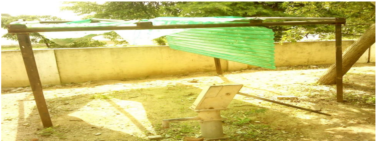
The temporary kitchen shed was used earlier by the SHGs in Jannaram Mandal now the meals is supplied by Akshaya Patra
