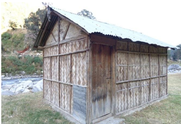
Kitchen Shed without ventilation
