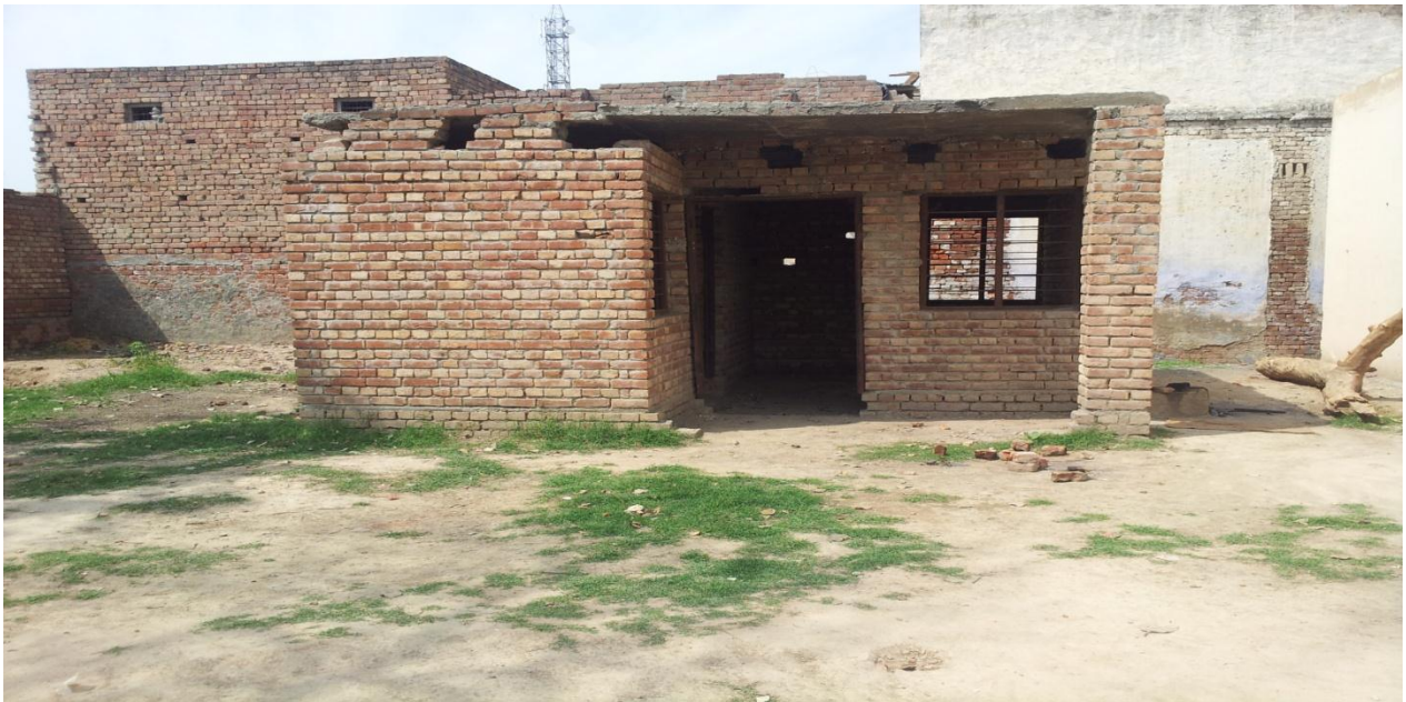
Incomplete kitchen cum store at Primary school Teek at Kaithal
